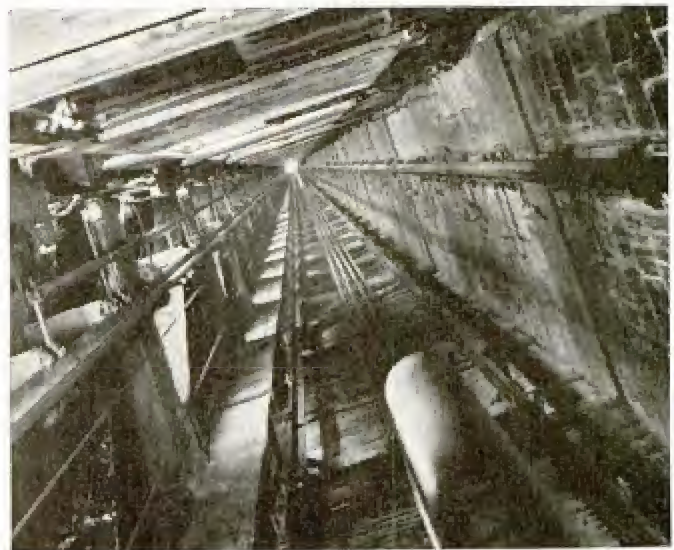
Looking down one of the 800-foot elevator shafts in the 70-story RCA tower. These elevators travel at 1,400 feet per minute
